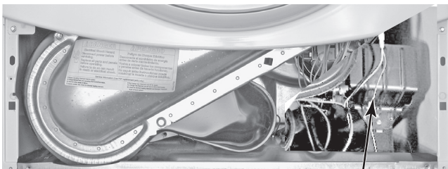
High-Limit Thermostat, Thermal Cutoff, & Heater Area
