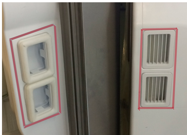
FIGURE 2: Foamed-In IM Duct Heater Locations
